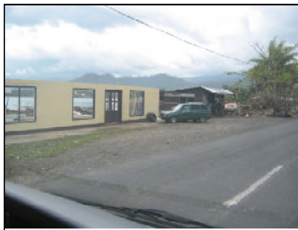
Family home damaged by Cyclone Heta
